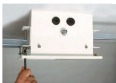
Adjust to ensure ceiling integrity
