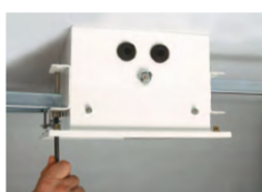
Adjust to ensure ceiling integrity
